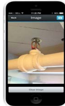
Photo of Defect
